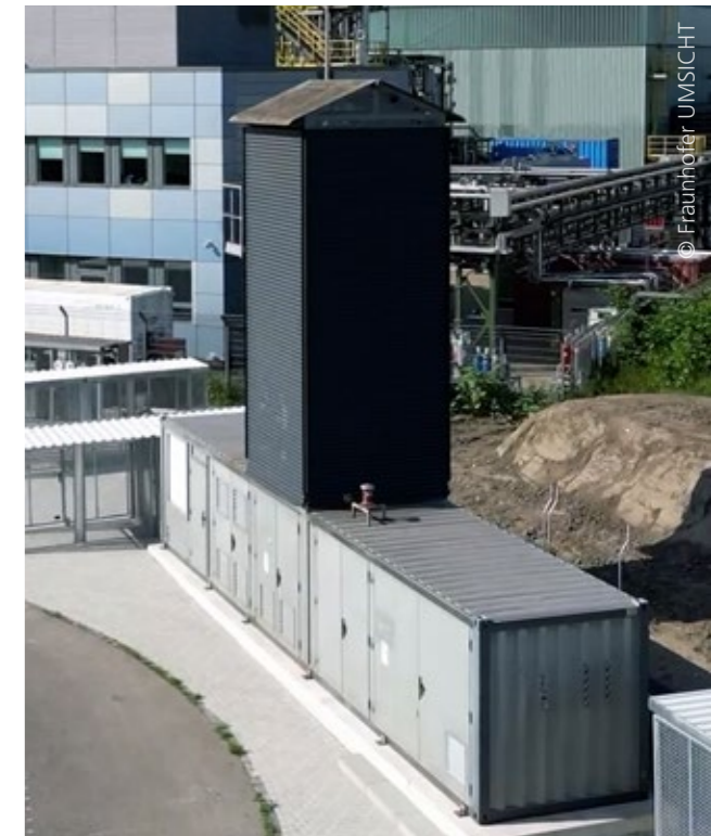
Methanol plant for the conversion of carbon-rich gases, developed at Fraunhofer UMSICHT as part of the Carbon2Chem® project
