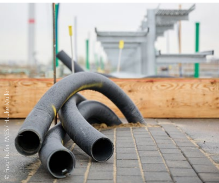
Construction of the Hydrogen Lab Bremerhaven in the immediate vicinity of the 8 MW offshore turbine.
