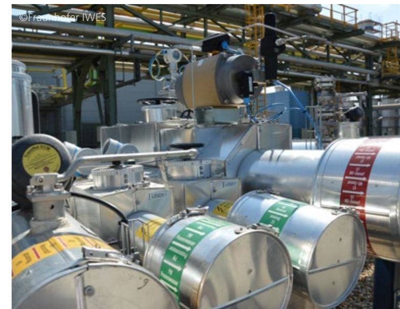
The Hydrogen Lab Leuna is already in operation.
