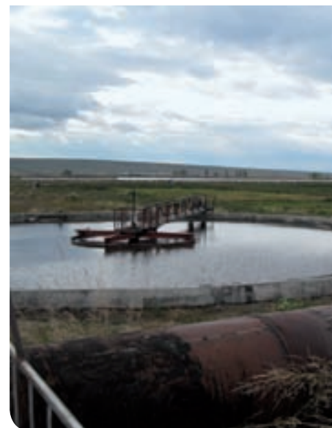
Room for improvement: Researchers want to boost the effectiveness of the wastewater treatment plant.
